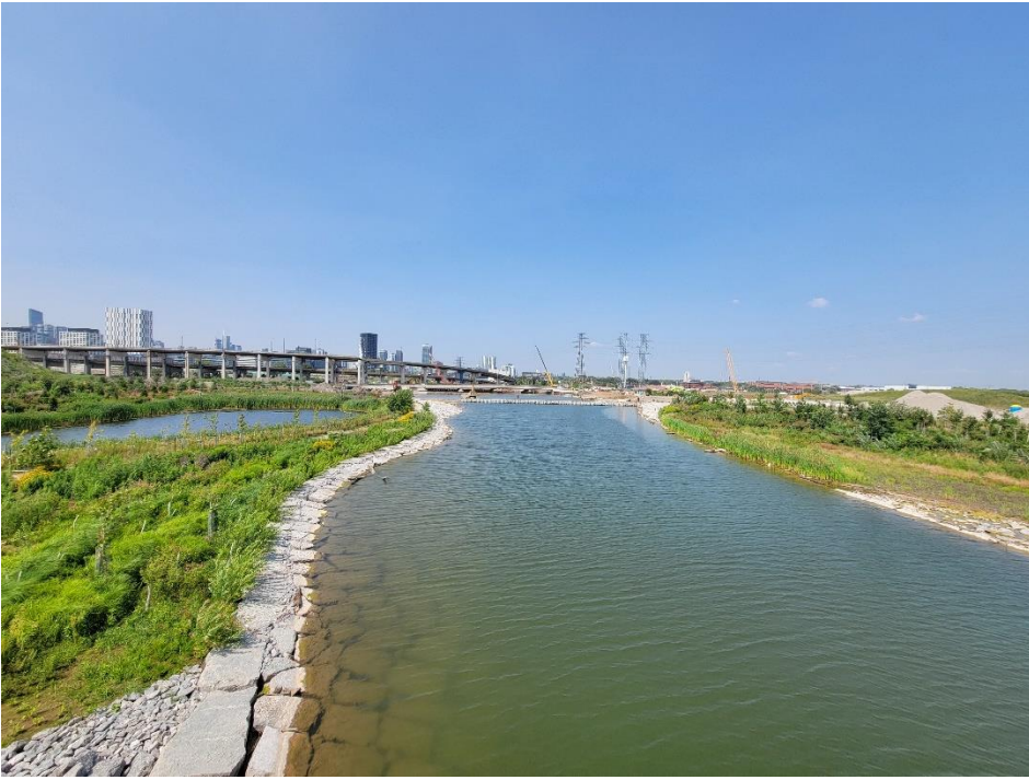
Looking north from the Commissioners Street Bridge, you can see the cutoff wall that is separating the new river valley from the existing Don River and Keating Channel. It will be removed by the end of the year.
