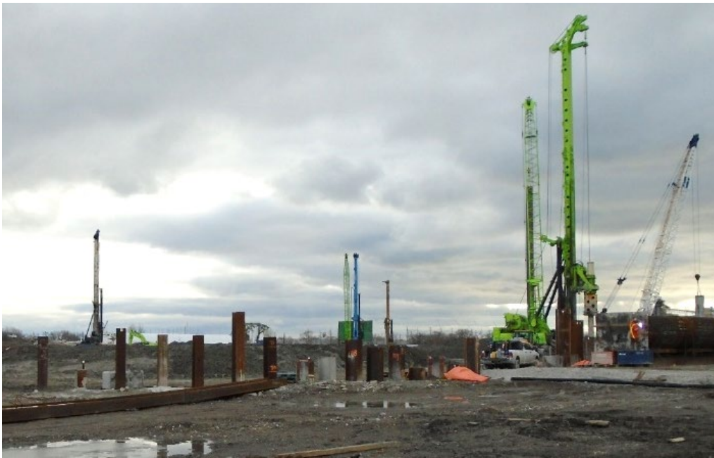
Above: Cut-off wall construction along the perimeter of the future river valley south of Commissioners Street just west of Don Roadway.
