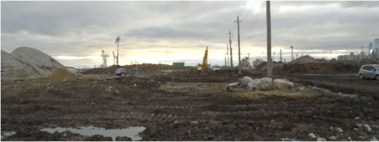
Above: Preparing for excavation in the future river valley north of Commissioners Street and west of Don Roadway.
