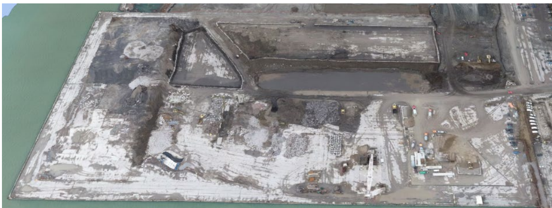
Above: Soil stockpile area on the site of the former Marine Terminal 35 building.
